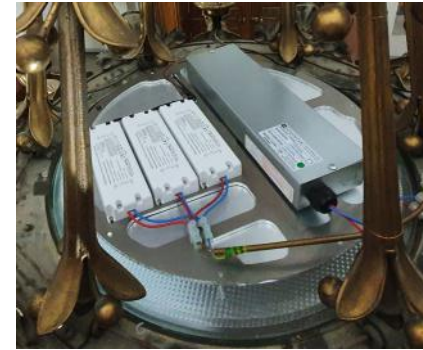
Up-Graded Chandelier with bespoke contemporary LED components including separate, battery-powered Emergency Lighting
