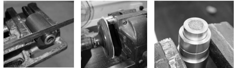
A uniquely-devised set of equipment and techniques enabled the repair of even severely-damaged Pmma fibre bundles—and all this in situ.
